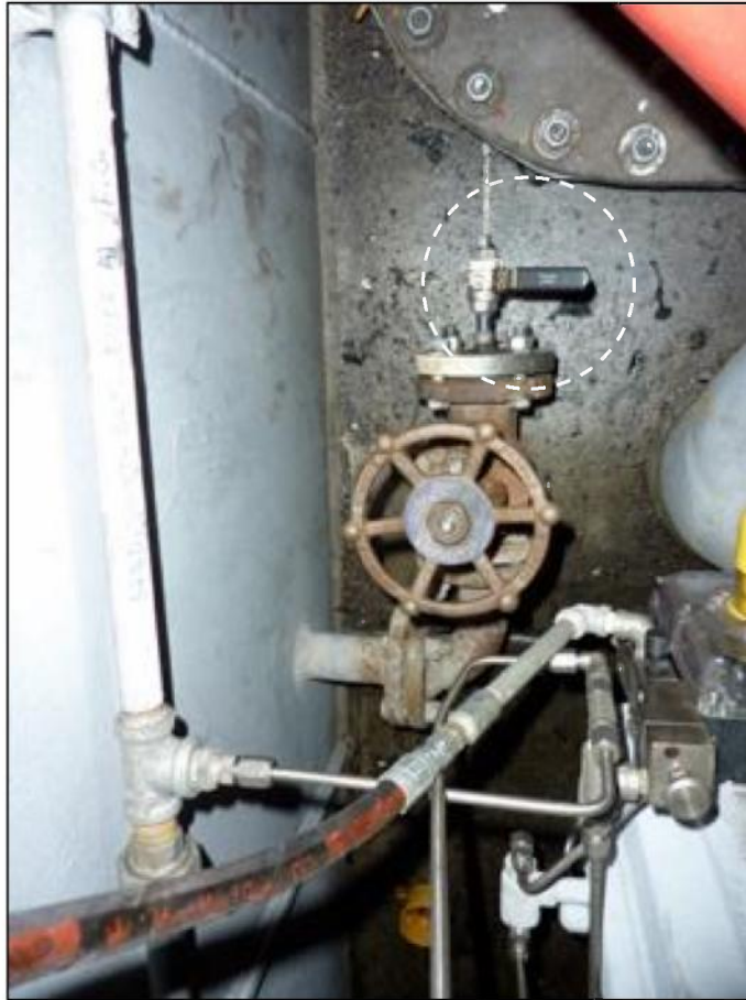
Photo 2 - No. 1 Day Tank Stbd Drain
