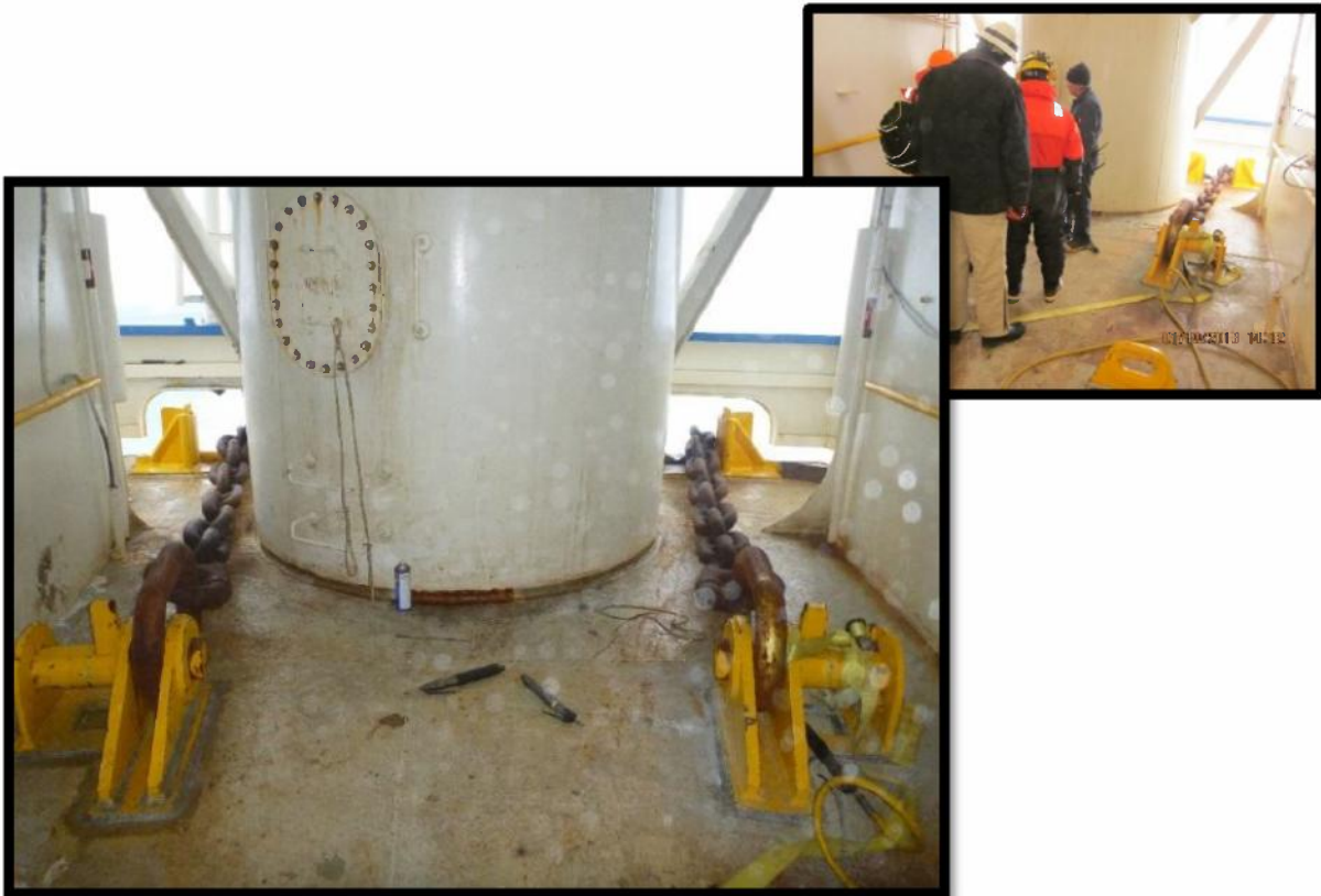
Figure 49: Photo of towing bridle connections to Smit Brackets (USCG Photo)
