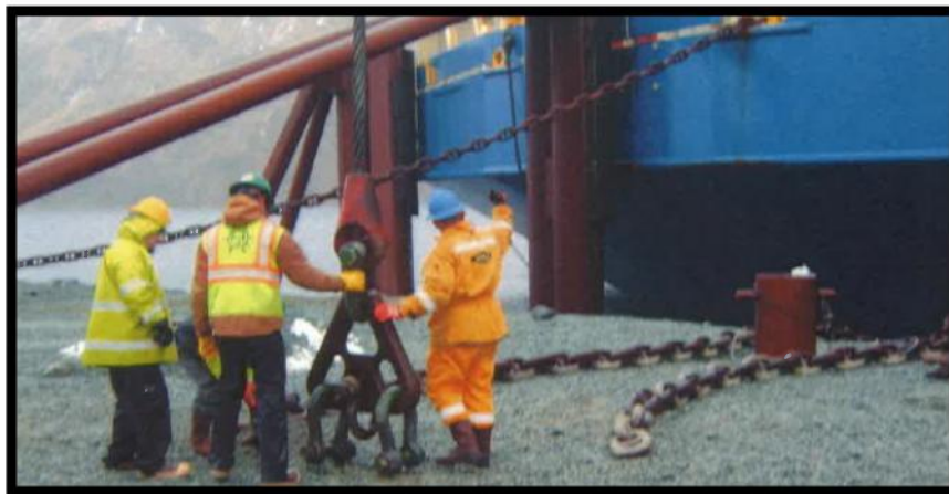
Figure 14: Preparing to Connect the Towing Plate to the Bridle Legs (Photo courtesy of GL Noble Denton, Mr. █████)
