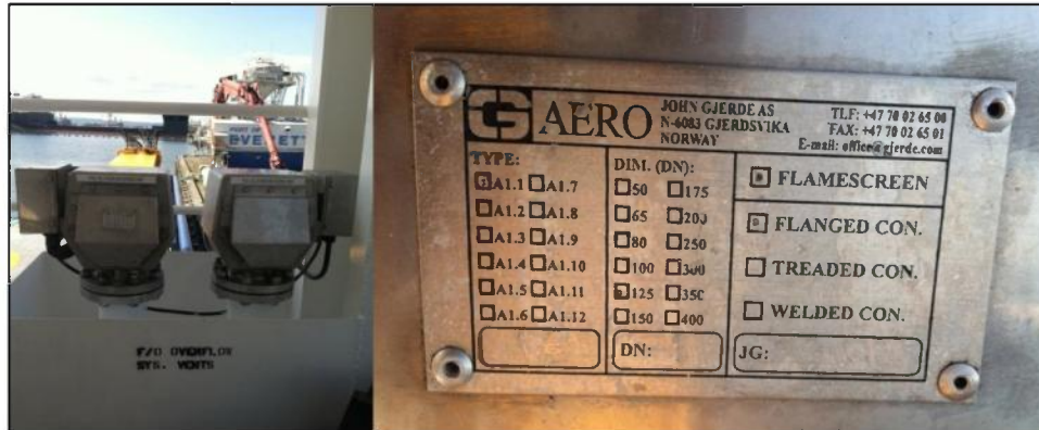
Photo 4 - Fuel Oil Overflow Vent (Typical)
