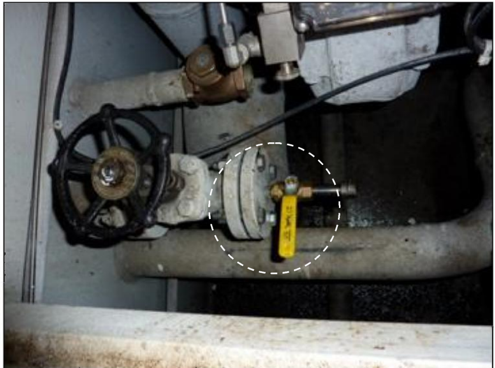
Photo 1 - Starboard Settling Tank Drain
